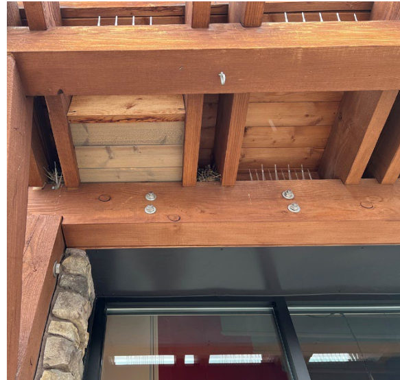
Figure 6. Bird spikes on a wooden beam. Note the nest in the middle of the image where spikes were not placed.
