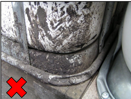
IBC is soiled with dirt
